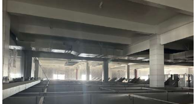
Figure 11: Equipment installed at the high-tech facility
